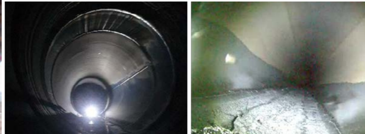
Inspection of the inside of pipelines at the Ulsan CLX of SK Innovation (robotic snake)
