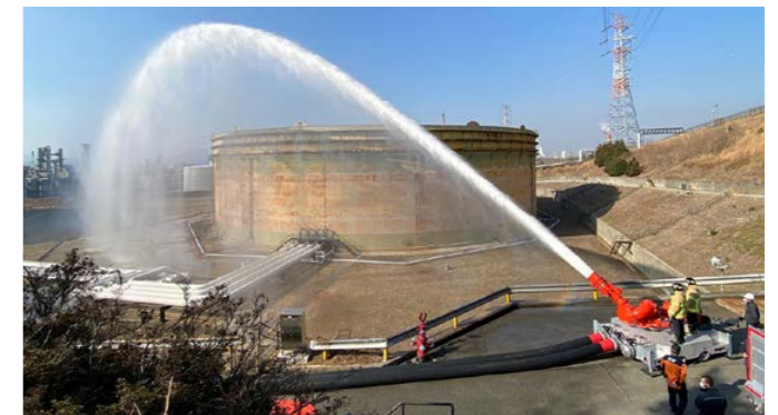
For the first time in Korea, SK Innovation has implemented a “high-capacity fire extinguisher” to swiftly extinguish fires in the large tanks within the crude oil storage area of Ulsan Complex.
